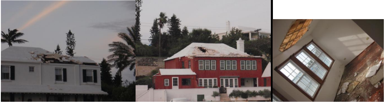
Figure 4: Roof damage at Pitts Bay Road, Hamilton, Pembroke
